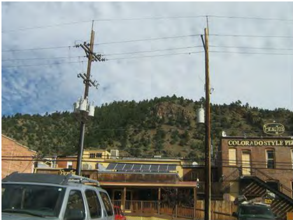
Photo 4. View of typical pole mounted transformers found throughout the project vicinity. No pole mounted transformers were found on the Site.
